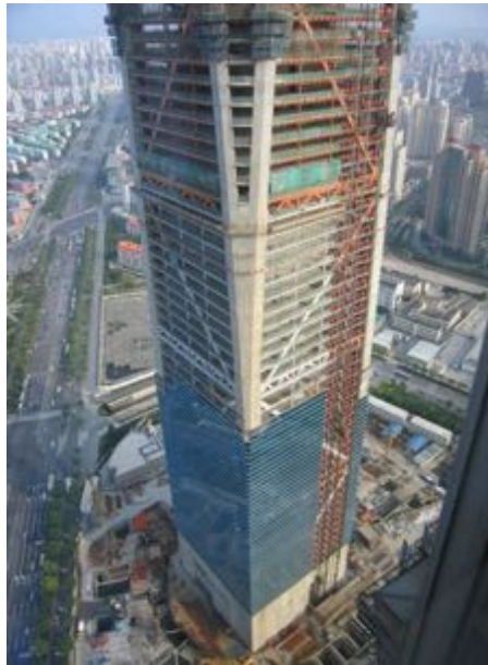
Belt and truss systems
